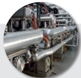
Water treatment supply
